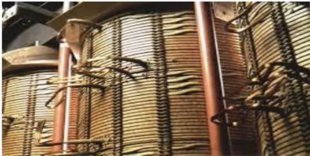
Figure 2.14 Transformer Windings Wrapped in Solid Insulation
