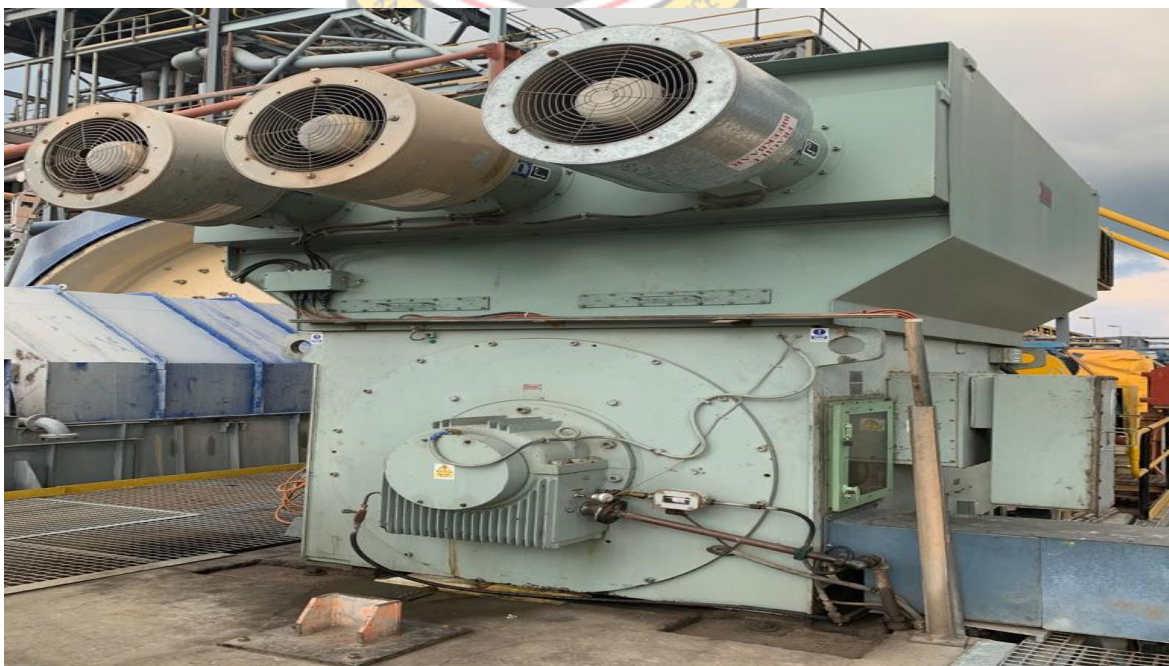
Fig. 3.1 Non-drive Side of the SAG Mill Motor
