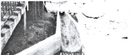
Construction of drains and a retaining wall at Asem in the Kumasi Metropolis of the Ashanti Region. Work is about 45 per cent complete.
