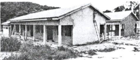
Construction and furnishing of a six-unit classroom block at Manso Zongo in the Amenfi Central District of the Western Region. Project is about 65% complete.
