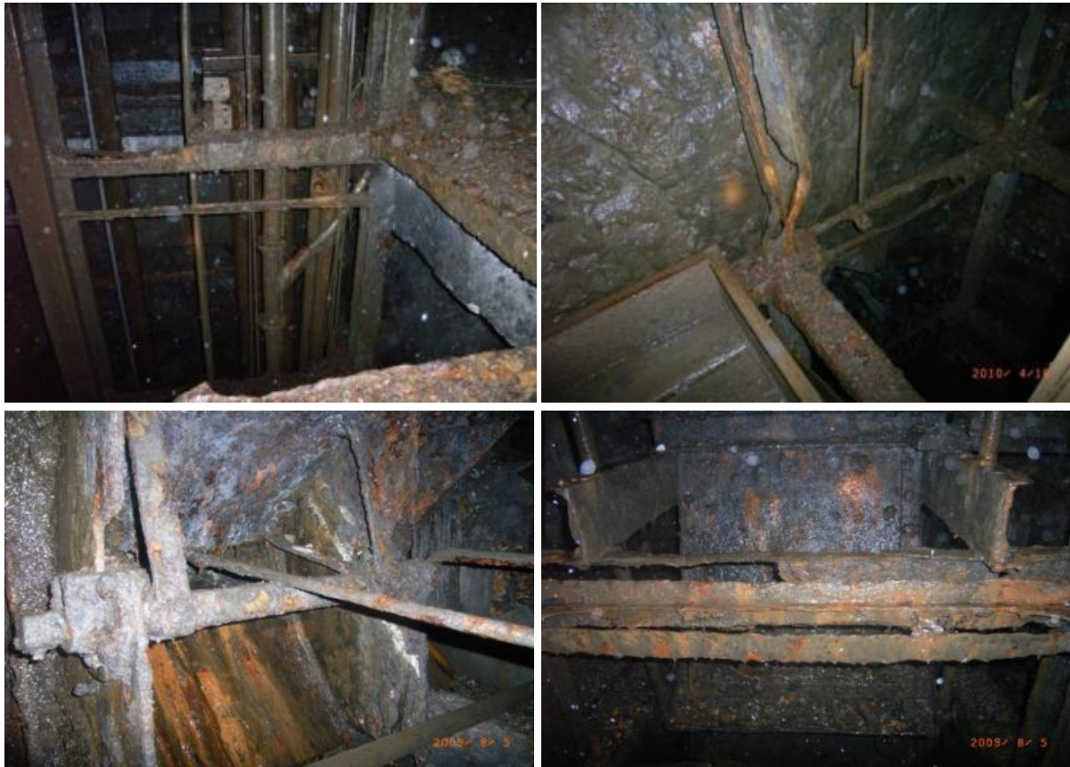
Figure 3: Condition of Shaft Infrastructure
