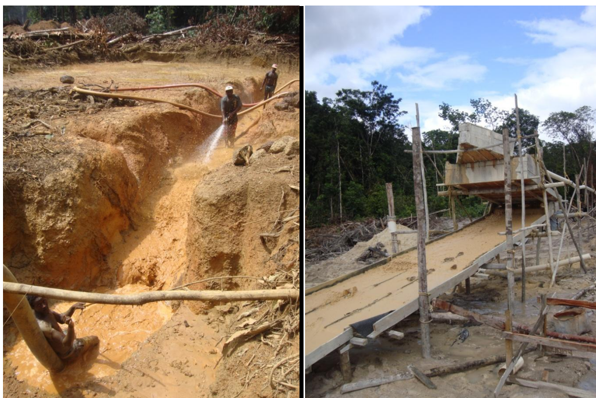
Left: Land dredgers channelling material to the pump man. Right: Typical sluice box
